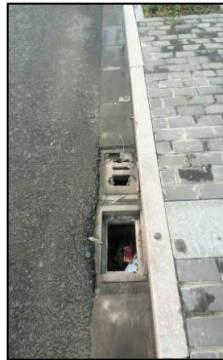
Manhole Cover Theft
